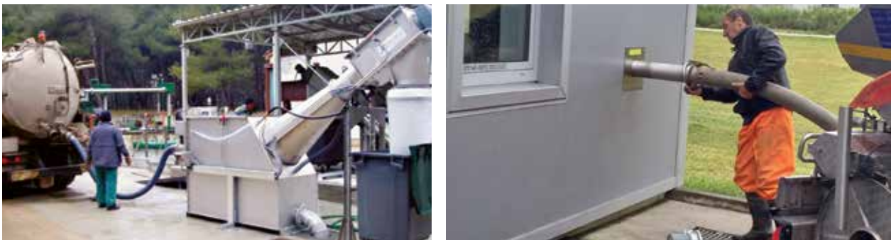
Figure 64: Typical photographs of the septage receiving station
